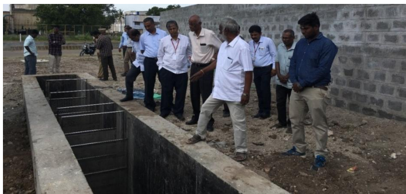
Newly established Sewage Treatment Plant
